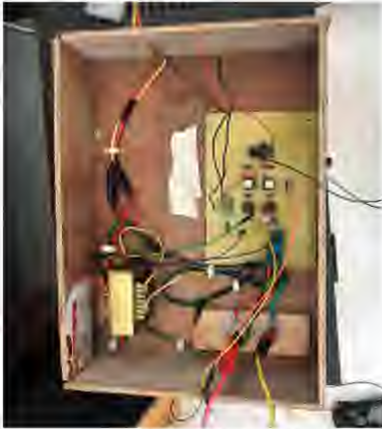
Fig 13: Circuit Setup of SEM
